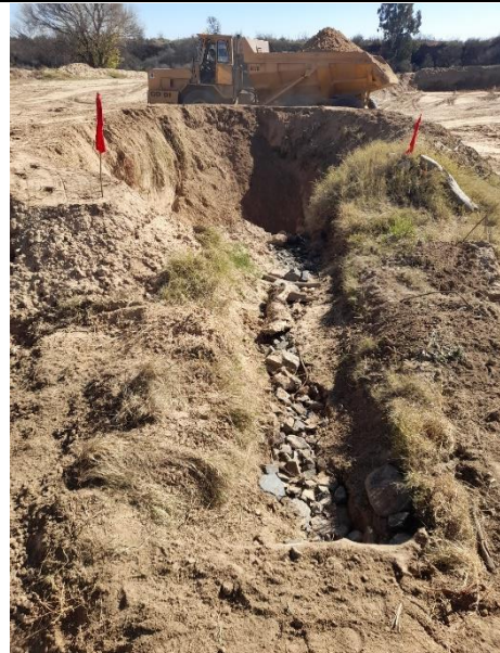
Drain to contain the runoff water from the washing plant
