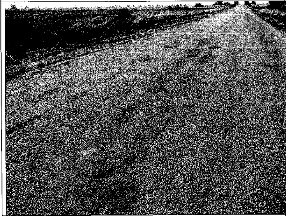
@ km 2.1 Surface Failure and Aggregate Loss is present for long sections of S171.
