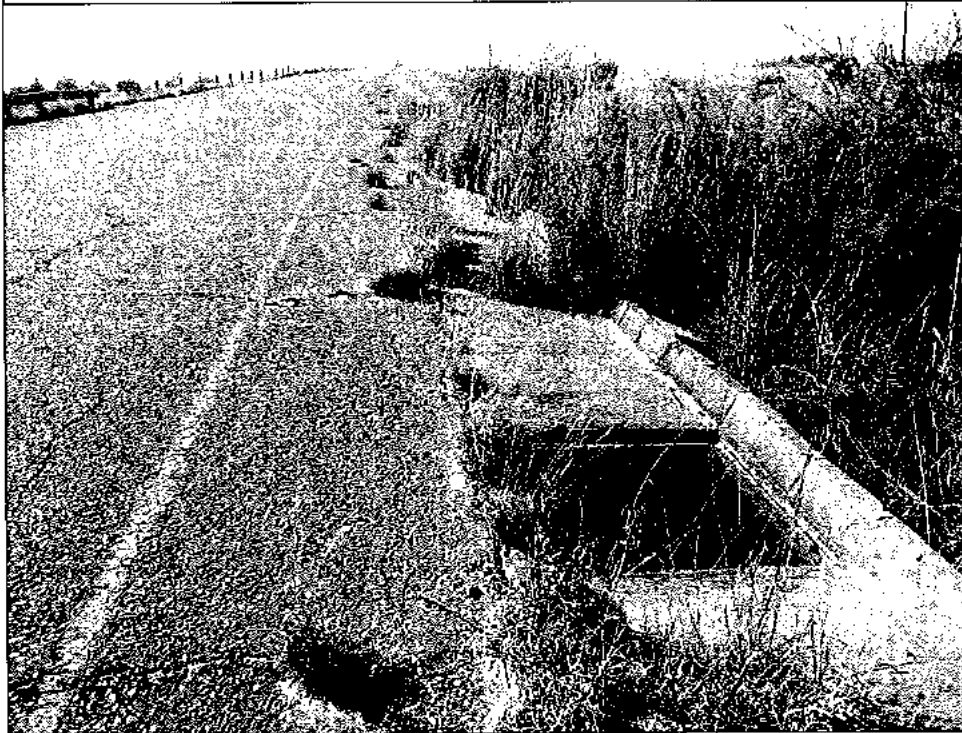
@ km 1.3 Missing storm water grid.
