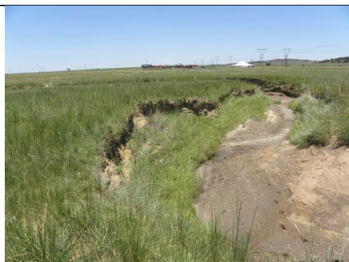
Photo 8: Portion of channel exposed to bank erosion
