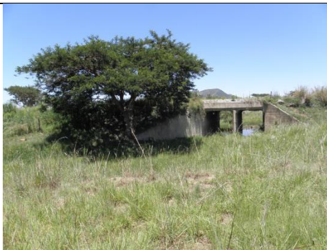
Photo 5: Culvert obstruction the natural flow of water
