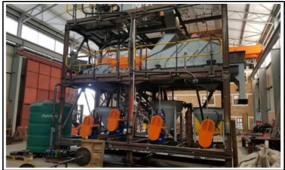
Figure 5: Image showing a typical DMS plant for producing spodumene concentrate (image obtained from Namli Exploration and Mining (Pty) Ltd).
