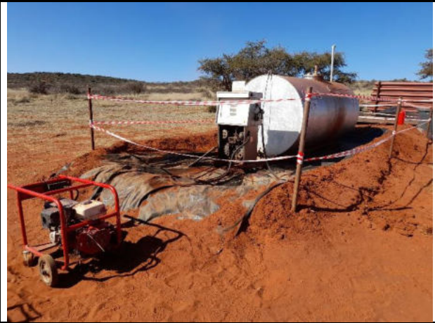
Diesel tank with bund. Generator to be placed in a drip tray
