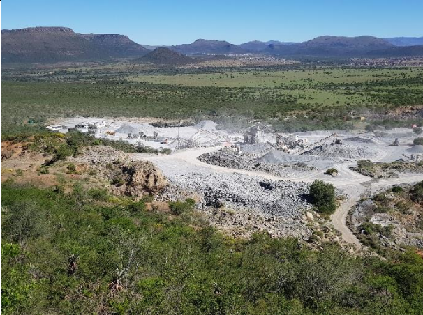
EXISTING PROCESSING PLANT OF QUEENSTOWN QUARRY WHERE THE MATERIAL WILL BE PROCESSED
