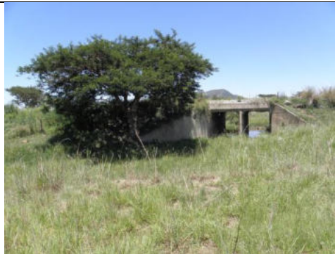
Photo 5: Culvert obstruction the natural flow of water
