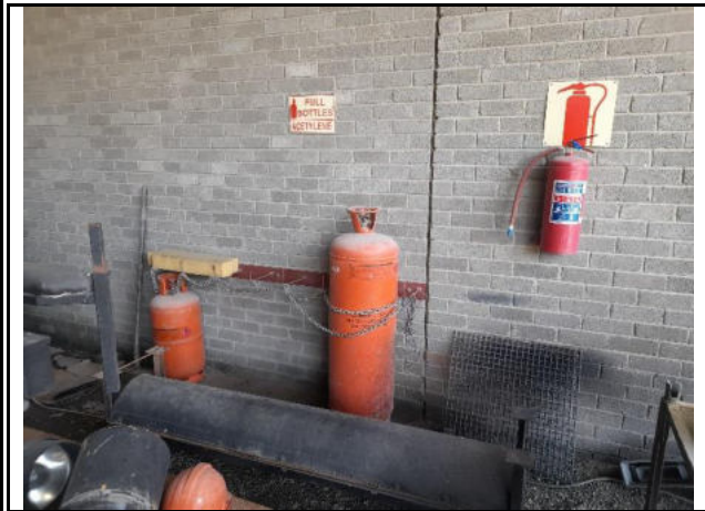
Gas storage area.
